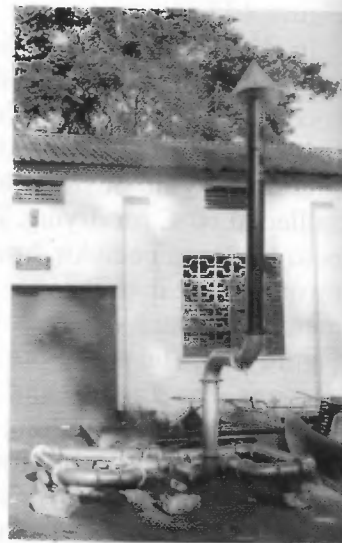
Figure 4.14 The heat exchanger used in the Otim dryer, Uganda.
