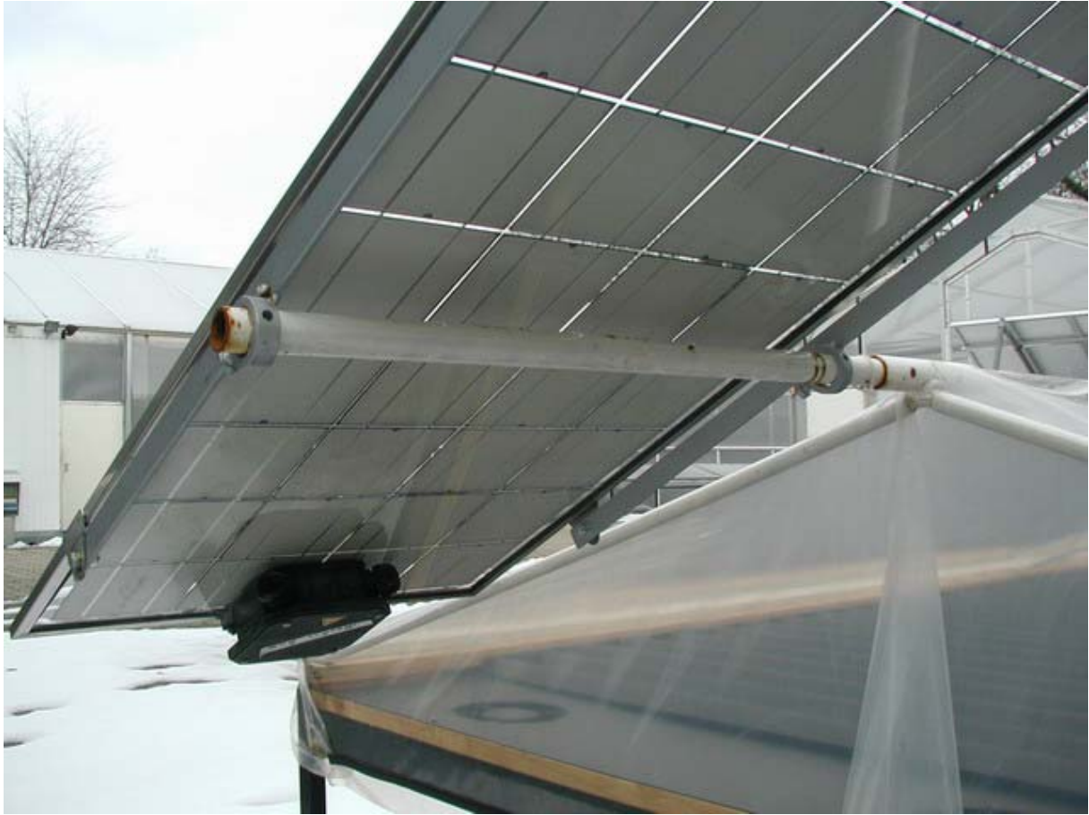
Fig: 49 shows the solar panel
